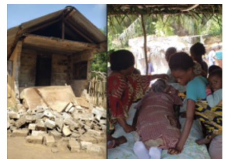
In mid-October 2022, 25 km from Lokutu, towards Lokumete, the wall of a worker's house collapsed, killing his wife.
